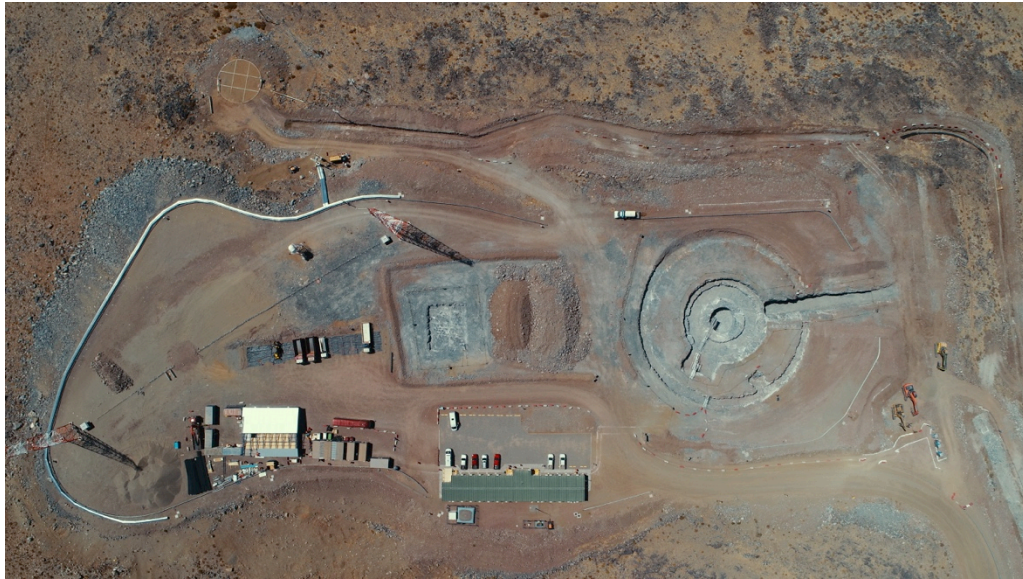
Figure 8. GMT site in March 2019, showing foundations for telescope pier and enclosure at right, and operations building at center. Courtesy of Giant Magellan Telescope – GMTO Corporation.
