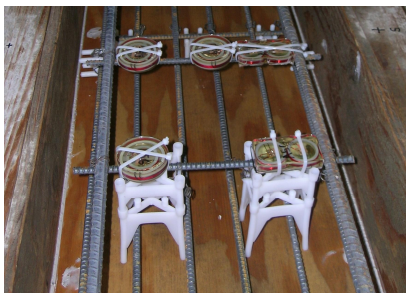
Figure 6: Plastic chairs were used to support the layers of reinforcement independently in Slabs 1 and 2.
